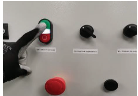
D Main motors will start and the indicator will illuminate (green light)
